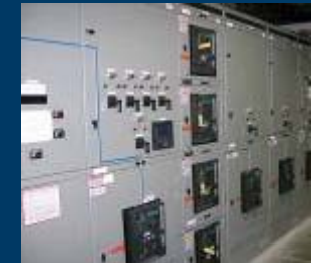
Data Center Innovation
